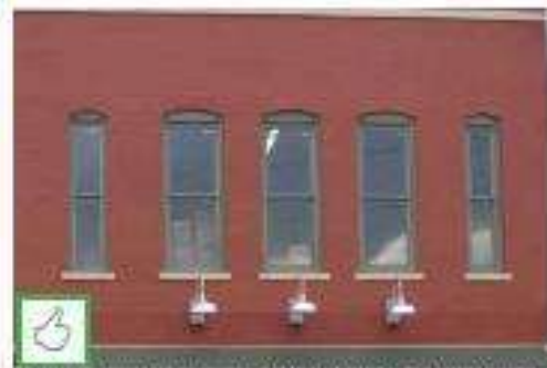
Commercial-grade replacement windows shall be sized appropriately to match the original masonry openings
