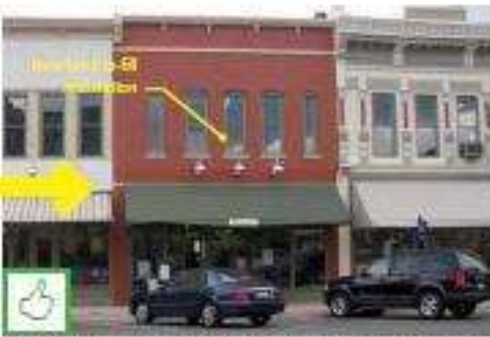
New brick in-fill was used to restore the upper story façade wall and window pattern and was painted to create a uniform façade (see photo to left).
