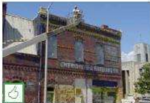
Original brick façade walls shall be restored where practicable by tuck-pointing and repointing the brick; this photo is during restoration.
