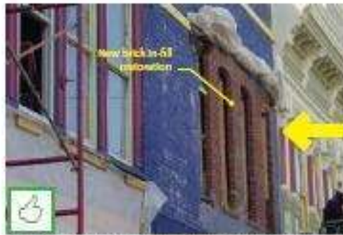
New brick in-fill is permitted where it is used to restore the original façade wall; note the appropriate upper story windows in this construction photo (see photo to right).
