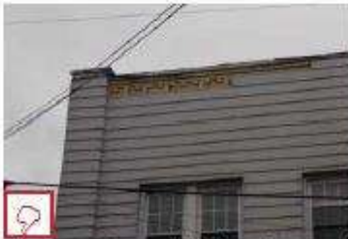
Covering or encapsulating original building façade walls is not permitted; note the original brick cornice detail beneath the siding.
