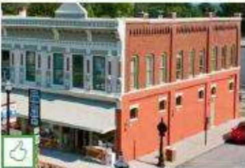
Restored brick façade walls may be either painted and/or remain natural; note this end wall has both applications.
